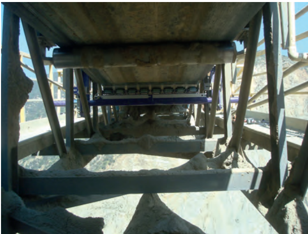
Figure 5. Secondary belt cleaners help to stop the spread of dust, limiting MSHA fine possibilities.
