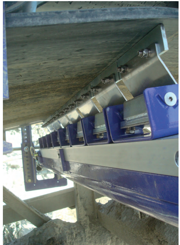
Figure 3. Secondary belt cleaners keep workers safe from the spread of harmful carryback.
